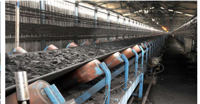
Coal Handling Plant
